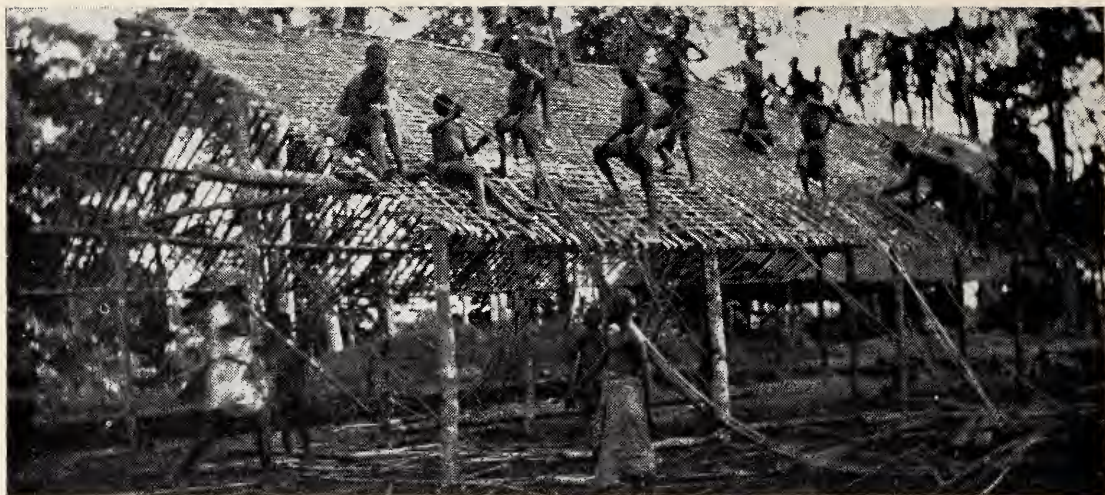
Native boys cooperate in the erection of a new school building prior to the opening of a new term. Mr. Schindler supervised the building.
